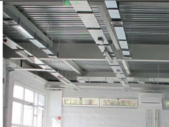
4. Natural and Artificial Lighting and Ventilation
